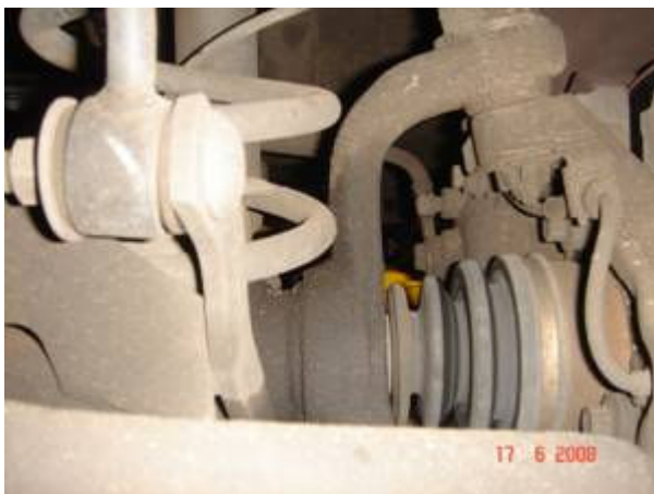
ZJ CV boot, the wet oil is an inner axle seal leak
